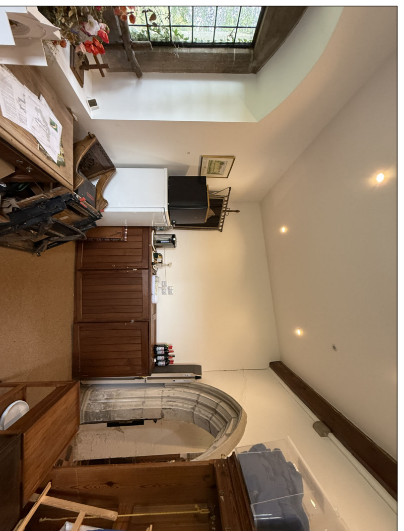
4 View from the West side of the westy, towards the East. This space is to be fully cleared to accommodate a new accessible WC and archive space. Chancel desk hooks and back rail to be retained and protected by the church FCC, for inclusion within the archive space.
