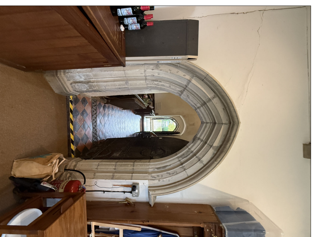
3 View from the westy to the South Entrance. Once the pew plinths are removed from a front of the westy door, a level threshold between spaces will be generated.
