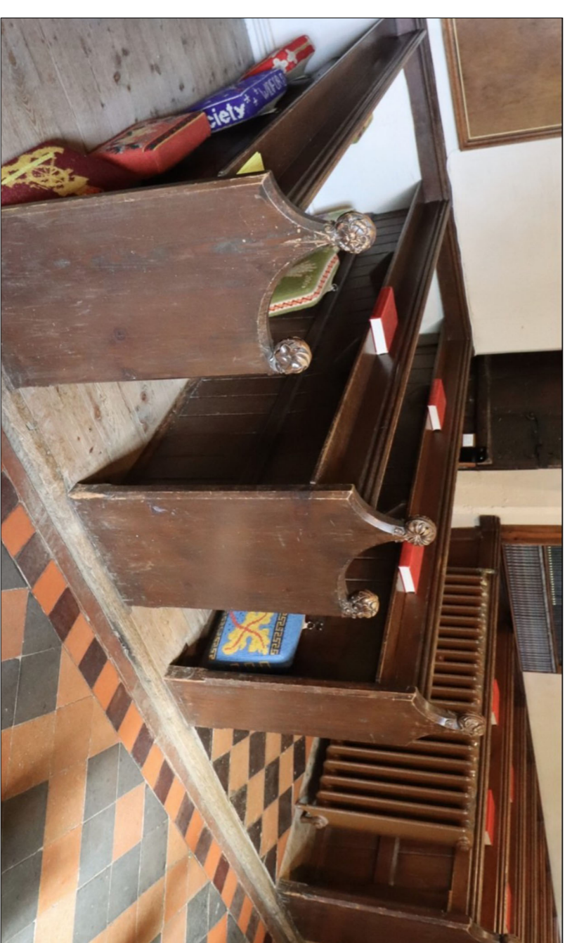
6 The pews are Victorian with very little ornament to them. The intention is for the doors of the new joined servery to have a bead-and-butt timber finial, which replicates the bead-and-butt timber visible in the existing pews.
